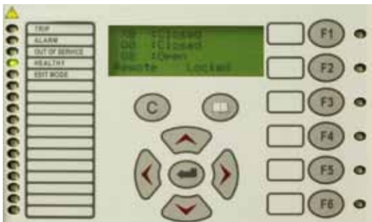
Local control panel with a text HMI
